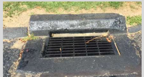
Metal storm water drains, stone curbs and other areas where excessive sealcoat was applied and can be easily identified can be good locations to collect samples.
